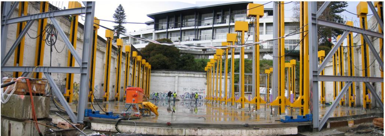
A system containing 36 synchronised jacks, ready to lift the first floor into position
